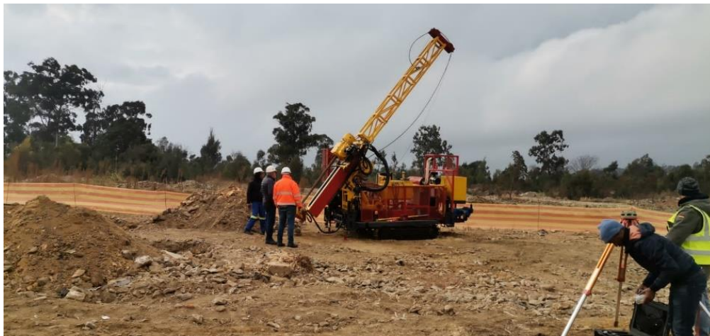
IMAGE 3: DRILL RIG SET-UP FOR THE FIRST DRILL-HOLE OF THE URANIUM EXPLORATION PROGRAM
